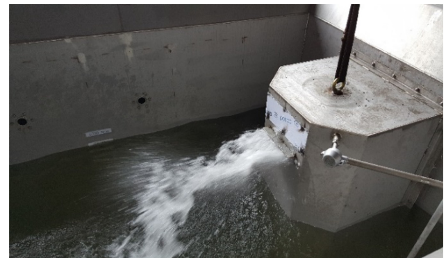
Fig. 6 Hot water pouring out of ejection gate in outer jacket
