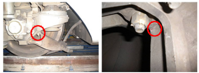
Fig. 1 Sand spray bracket and crack position of bracket
